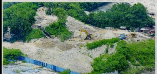
Illegal sand washing operators in Jalan Kelang Lama are back at it again despite Khalid ordering them to cease operations.
